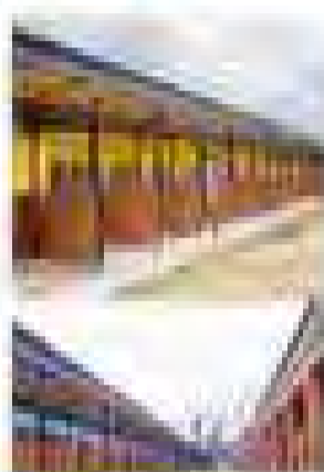
Construction of Ayetoro market with a total of 100 multi-purpose shops and 175 key clamp stalls
